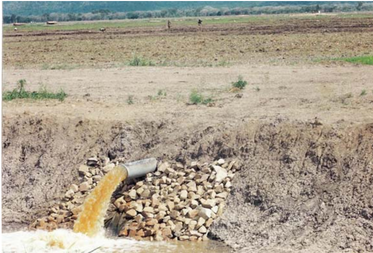
Photo 8.9 Full pipe discharging water from tertiary drain into main drain in Madibira despite other farmers needing water within the tertiary block. The discharge from the pipe is approximately 50 l/sec or two thirds the design inflow.
